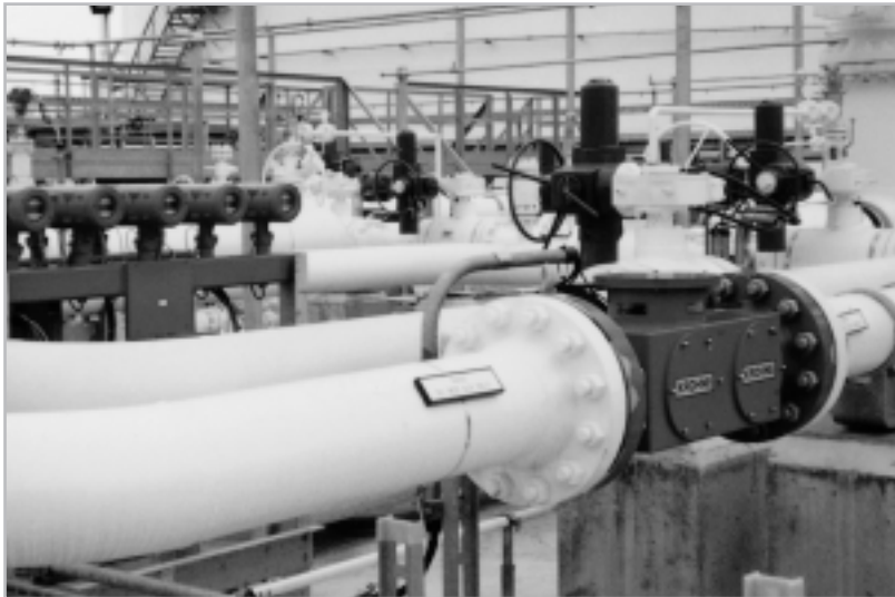
Fig. 29: Calibrated ALTOSONIC V ultrasonic volumetric meter with 5 measuring paths in a pumping station of the RRB pipeline
